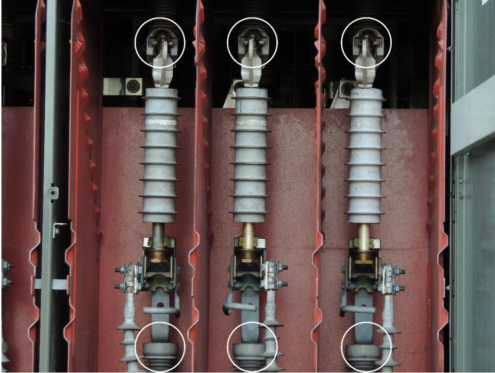
9. Upper and lower fuse insulators show signs of excessive contamination.
