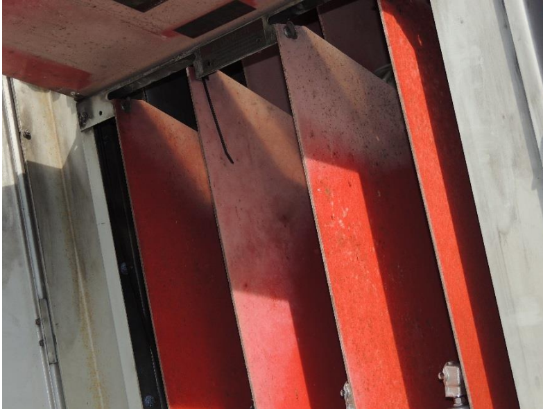
5a. Barrier boards are contaminated and discolored. One of the barrier boards is secured with a wire tie instead of an appropriate thumb screw.
