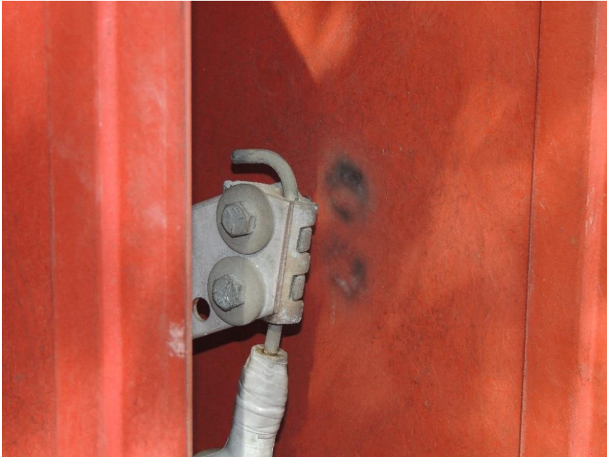
5c. Signs of electrical activity on the barrier board.
