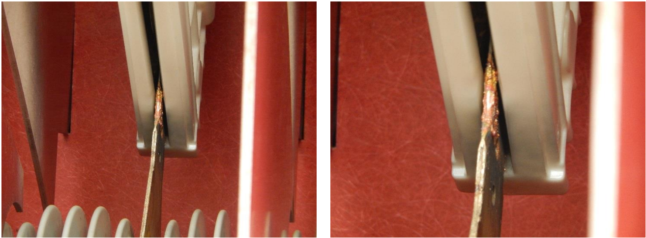
10a. Signs of arcing and melting at the disconnect blade.
