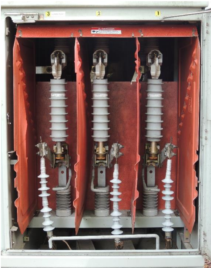
5b. Barrier boards at the center are bent.
