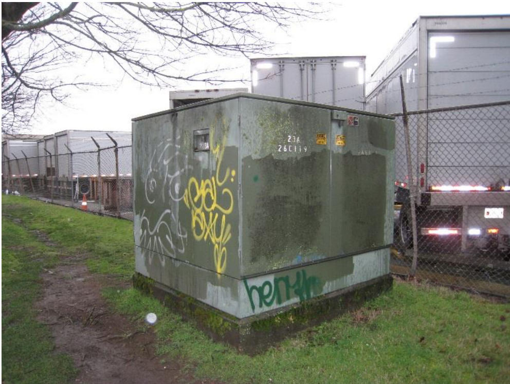
2b. Switch surface is covered with excessive moss and graffiti.
