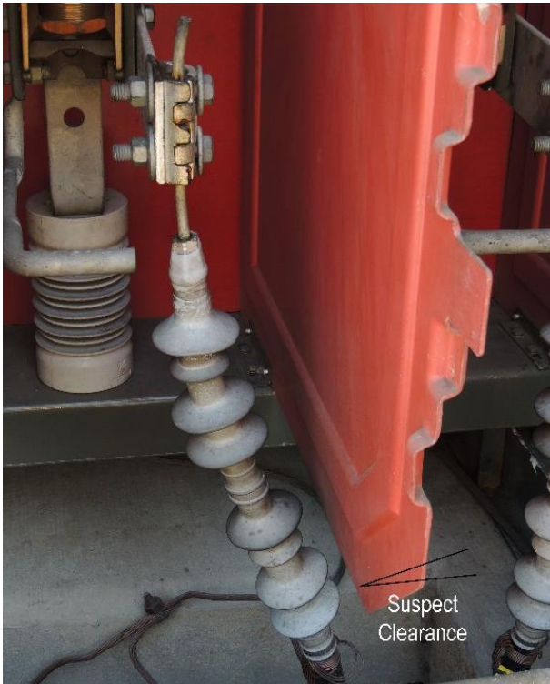
6d. Termination is too close to the barrier board.
