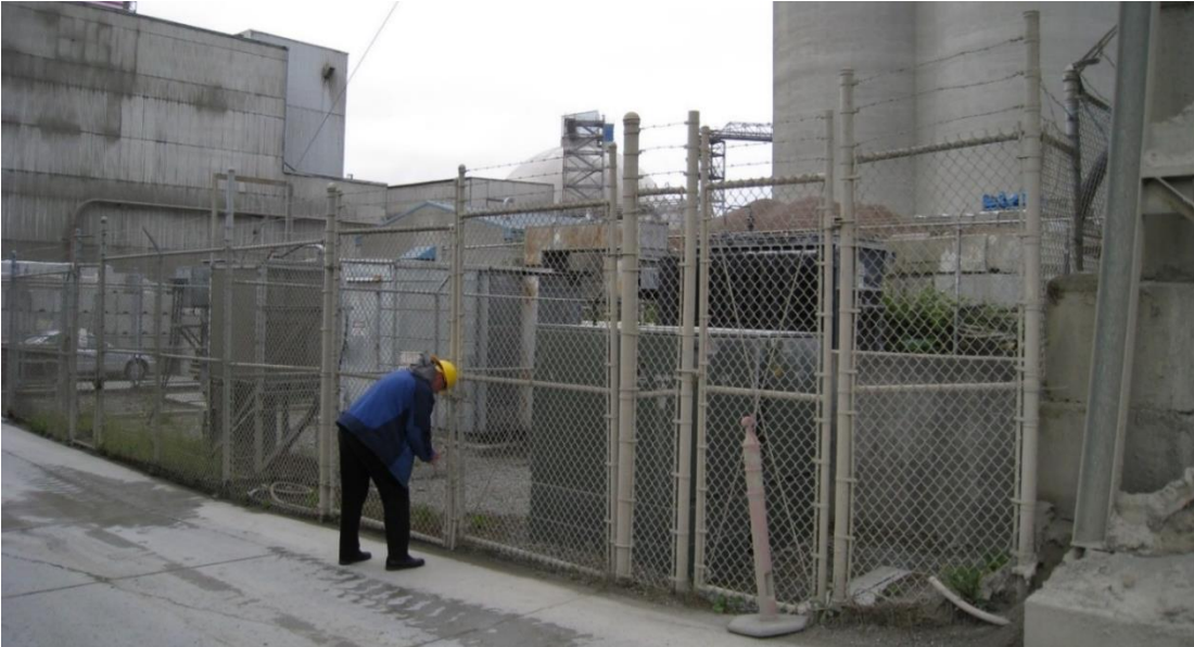
1a. Switch located inside customer's substation as shown.
