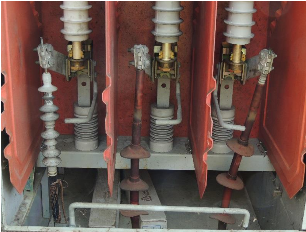
6b. Two terminations on the right side appear to be an older vintage. The termination skirts on the left termination extend far below the ground studs. The alignment of the termination skirts and the ground studs should be similar to one shown in photo 7.
