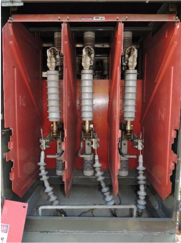
6c. Two terminations on the far left are bent and are pulling on the terminal pads. The termination on the right appears to be touching the concrete pad. The terminal pads are in the Standard position.
