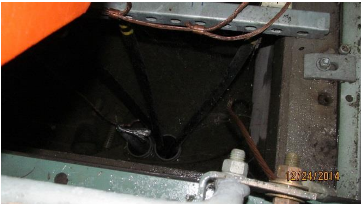
3b. Conduits are not sealed and a vapor barrier is not installed.
