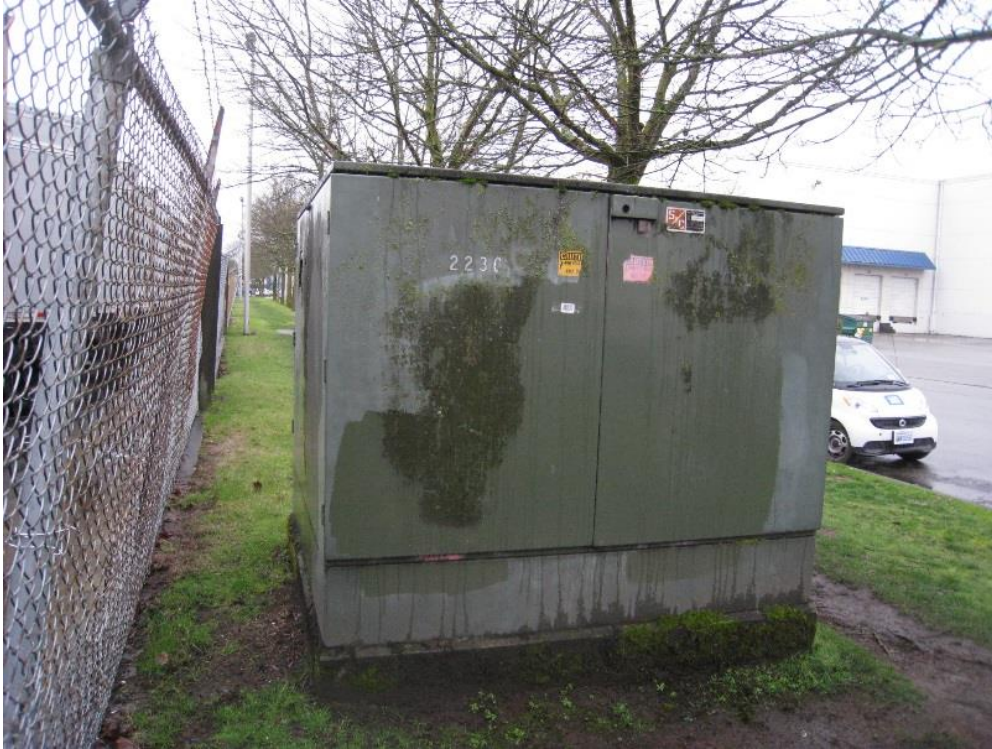
2a. Switch is missing danger and warning signs. The existing caution signs are outdated and damaged.
