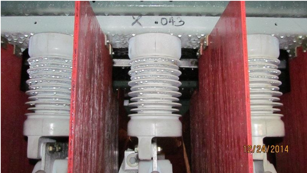
3a. Excessive condensation build up on the insulators and interior of the switch.
