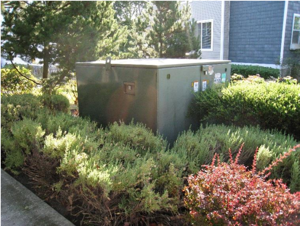
1c. Switch is not accessible due to excessive vegetation.
