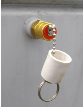
Figure 6.8.1 Pressure Relief Valve
