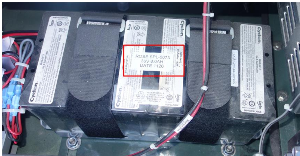
Figure C.1a. Remote Supervisory Battery Pack
