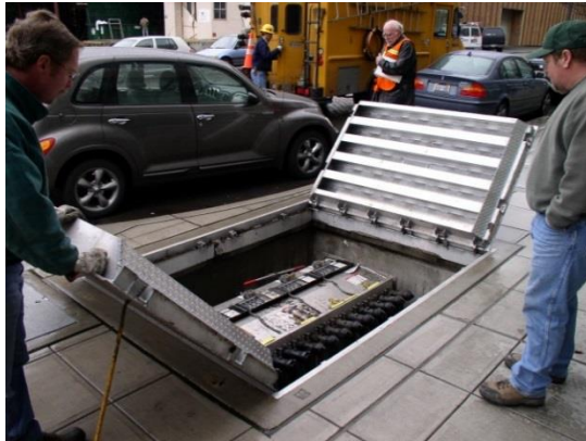
Figure 4.1.3. Switch in Wet, Subsurface Vault
