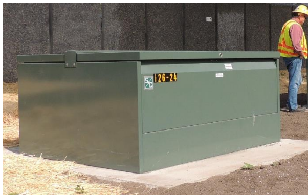
Figure 4.1.1. Manually Controlled Padmount-Style Switch
