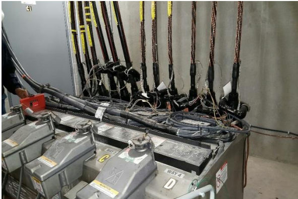
Figure 4.2.2a. Switch in In-Building Vault
