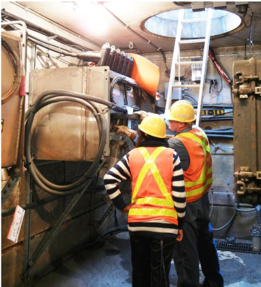
Figure 4.2.4a. Switch in Wet, Subsurface Vault
