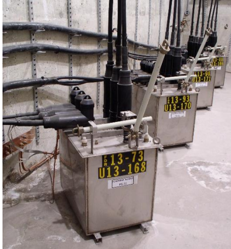
Figure 5. Puffer Pak Subsurface SF6 Switches
