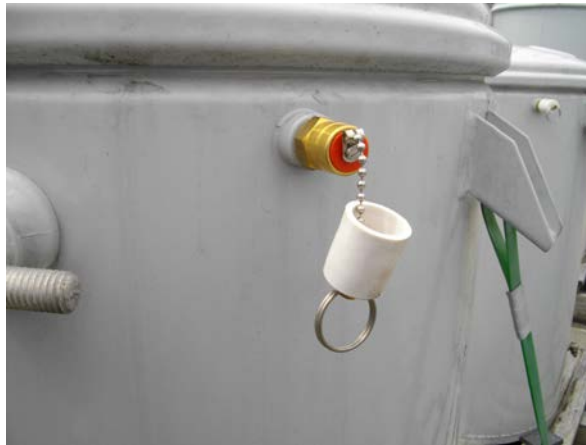
Figure 4.1. Transformer Pressure Relief Valve, Activated
