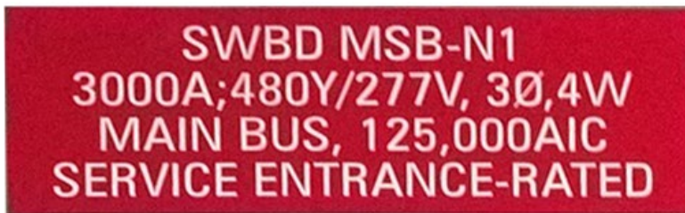
Figure 3.7. Example Placard for Dry Vault Service Entrance Buses
