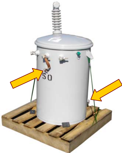
Figure 2 Overhead Transformer Ground Clamp Locations
