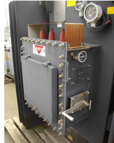
Figure 7.1, Bushing and Switch Chamber
