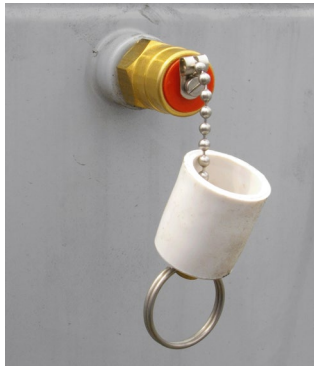
Figure 6.8. Pressure Relief Valve
