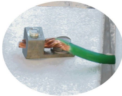
Figure 6b. Pole Ground Grounding
