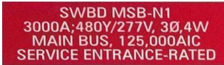
Figure 5d. Service Entrance Sign for Cable in Conduit Example
