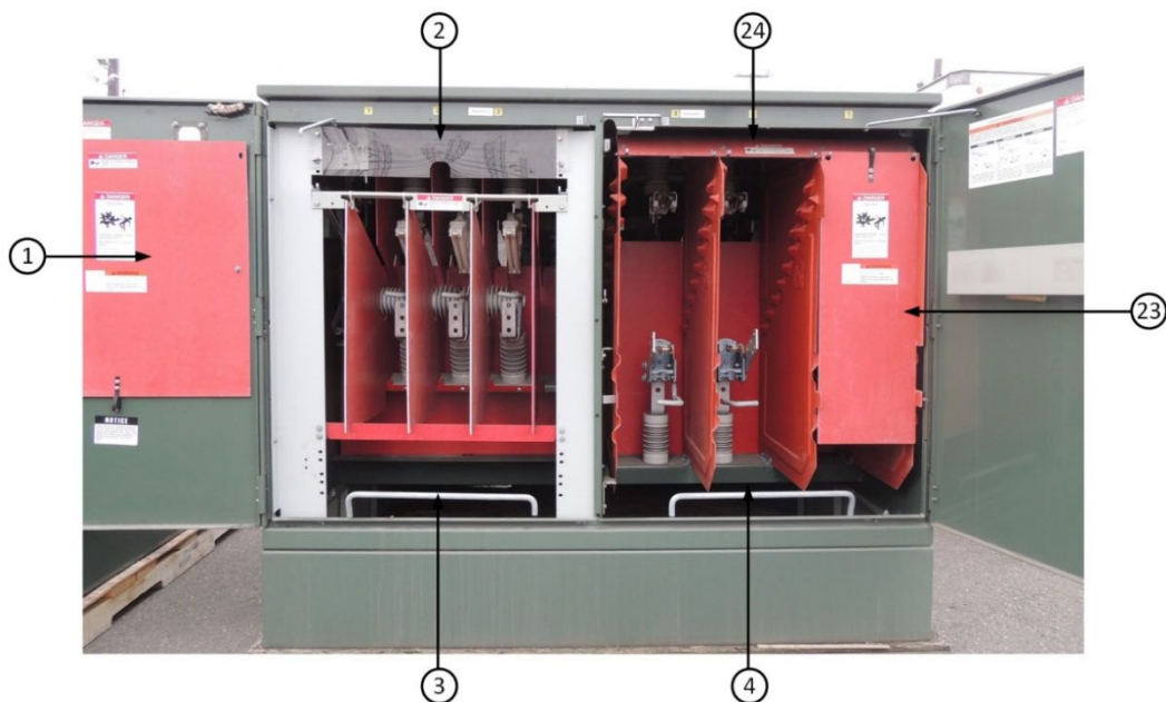
Figure 7c. PMH-11 Switchgear Compartments 3 and 4 Overall View
