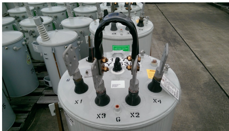
Figure 6.3b. Transformer with Jumper Connected to X2 and X3 Terminals
