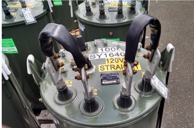
Figure 6.3.2b. Cut straight parallel-connected transformer with jumpers connected to X1 and X3 terminals and X2 and X4 terminals
