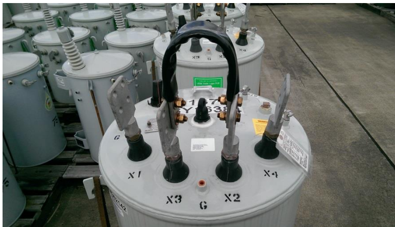
Figure 6.3.2a. Transformer with jumper connected to X2 and X3 terminals
