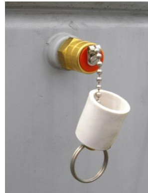
Figure 6.7 , Pressure relief valve
