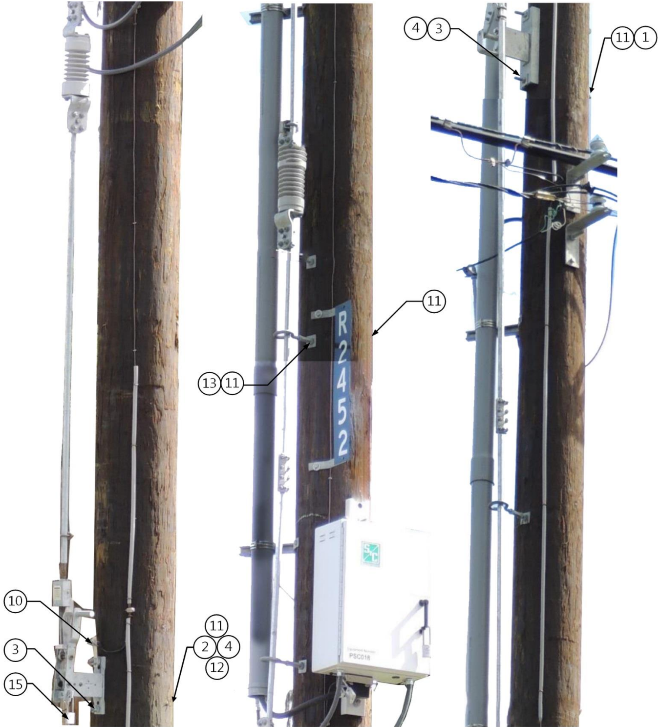
Figure 3c. Ground-Level Disconnect Handle Assembly
