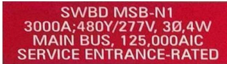
Figure 5c. Service Entrance Sign Example
