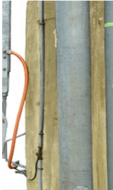
Figure 3.4 Switch Handle Grounding
